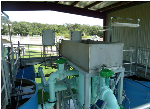
An influent flow splitting box evenly distributes flow to the treatment system
