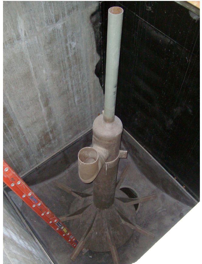
Concrete CF-64 cell prior to being charged with media.
