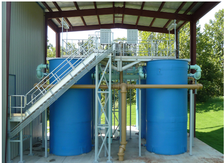
Six Model CF-64, 0.5 MGD average flow, 2.3 MGD peak flow phosphorus removal system at the Lincoln WWTP
