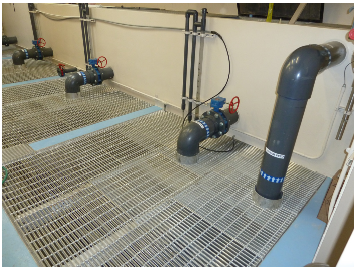
Convenient in-ground installation of the Blue PRO® filters in Georgetown.
