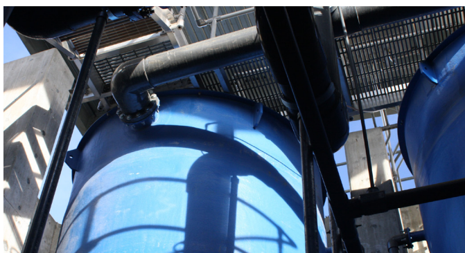
A view of the Centra-flo® filters from below
