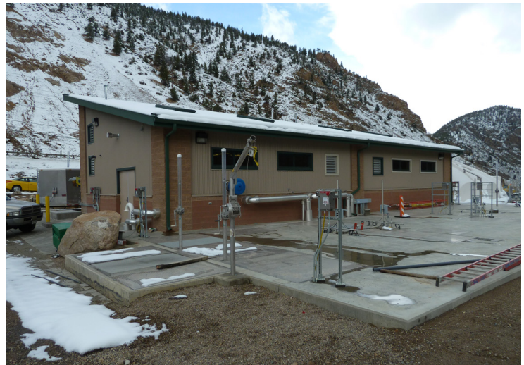
The building was erected during plant expansion and Blue PRO ® filter installation.
