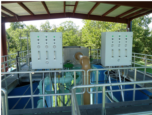
The Blue PRO® system air control panels
