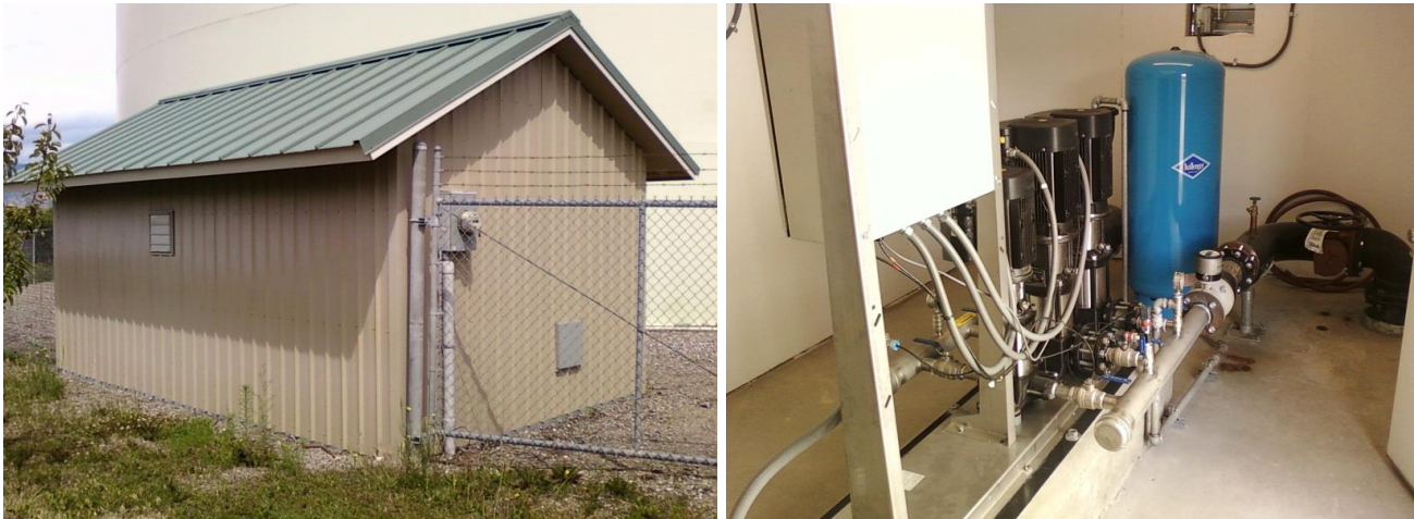
Photo 1-10 Vista Heights Booster Pump Station
