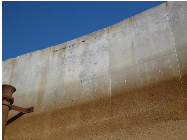
Photo 4: Rebar Corrosion at Top of Wall
