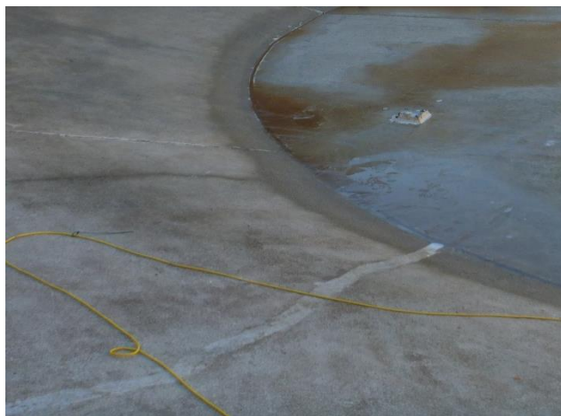
Photo 9: Previously-Sealed Floor Crack
