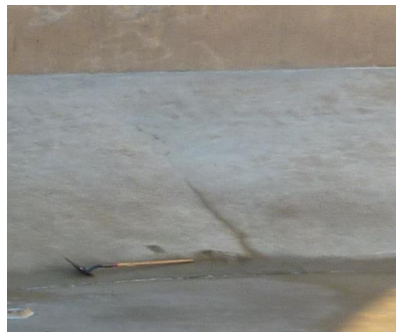
Photo 10: Actively Leaking Floor Crack
