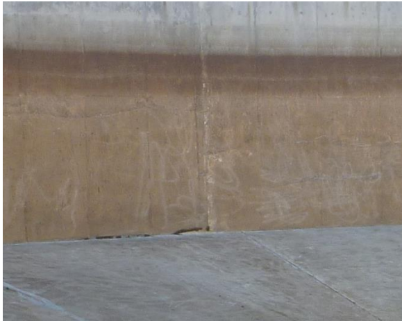
Photo 5: Area of Potential Rebar Corrosion
