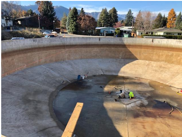
Photo 3: Rust Sediment at Tank Floor
