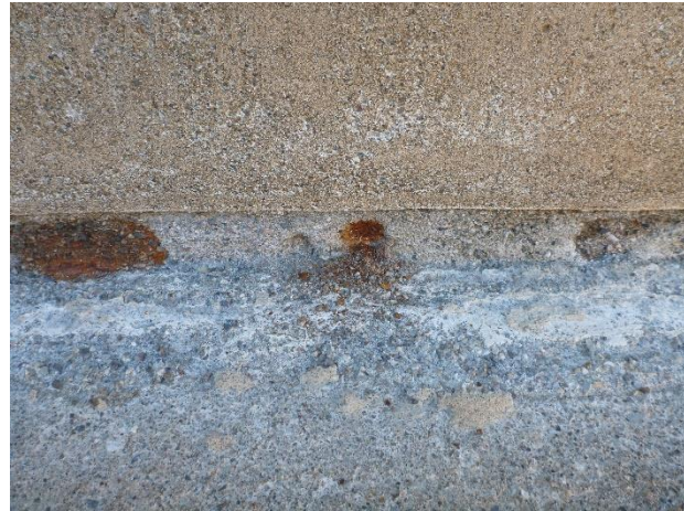
Photo 6: Potential Rebar Corrosion
