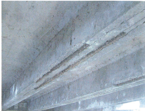
Photo 1 - Existing Girder Deterioration
